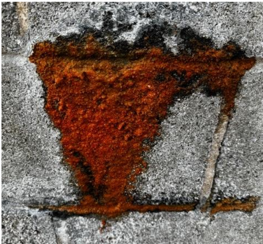
Concerning chemicals are protruding through the retaining wall along 21 st PL.
