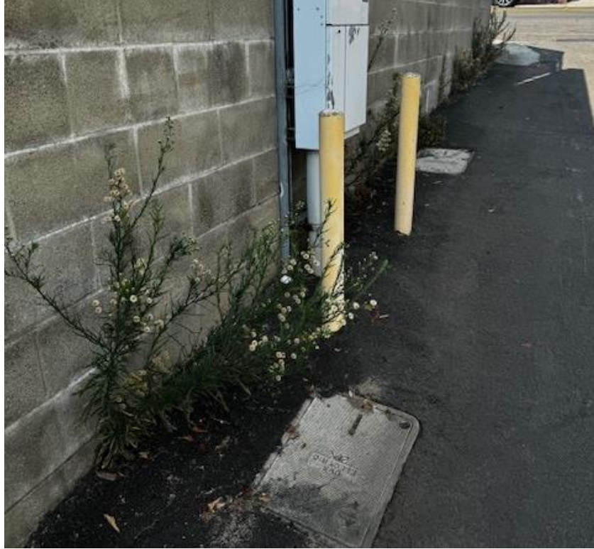
Weeds building up around the 2121 Highland property, creating localized problems for neighboring property owners.
