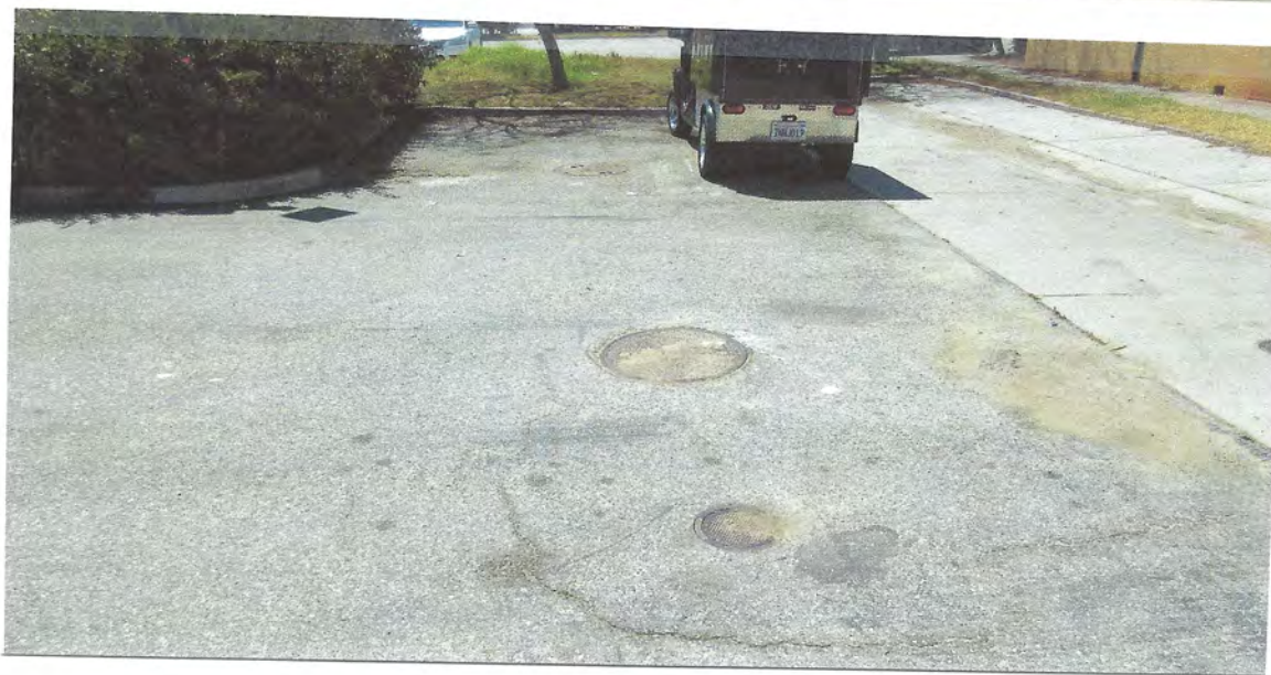
Photographs 5, 6 and 7 - View of water-service piping on the south edge of the site's parking lot; view of non-hazardous refuse bins seen in Photograph 4; and view of a multi-chamber "grease trap", in nearby area of the site's parking lot.
