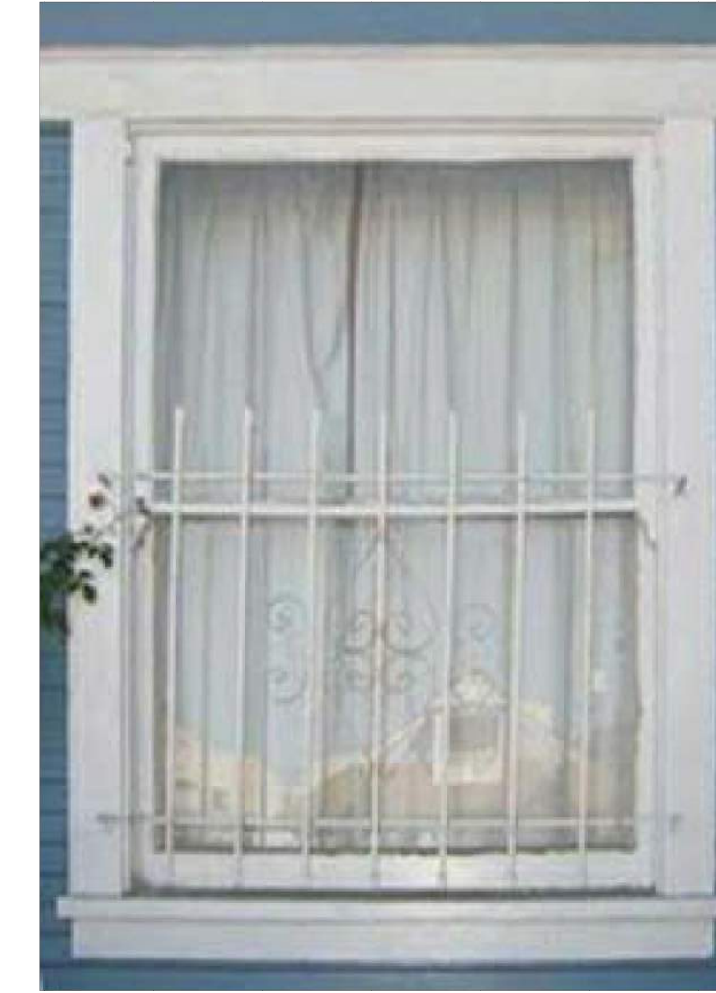
IMAGE: 849 SAN VICENTE WOOD WINDOW & TRIM SAMPLE. IMAGE OF HISTORICAL WINDOW AND SURROUNDS TO REMAIN
