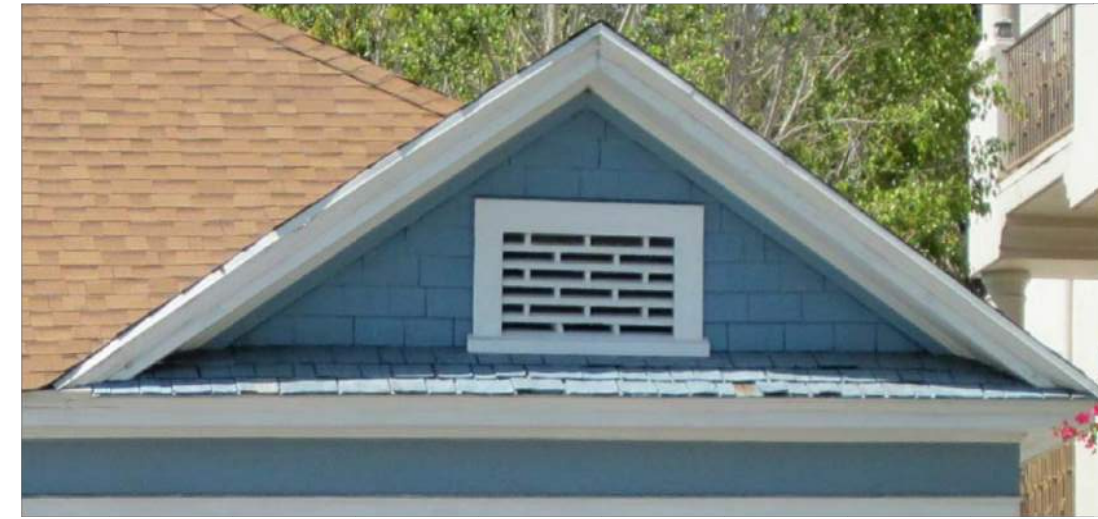
IMAGE: 849 SAN VICENTE. SAMPLE IMAGE OF GABLE VENT DETAILING TO BE RETAINED
