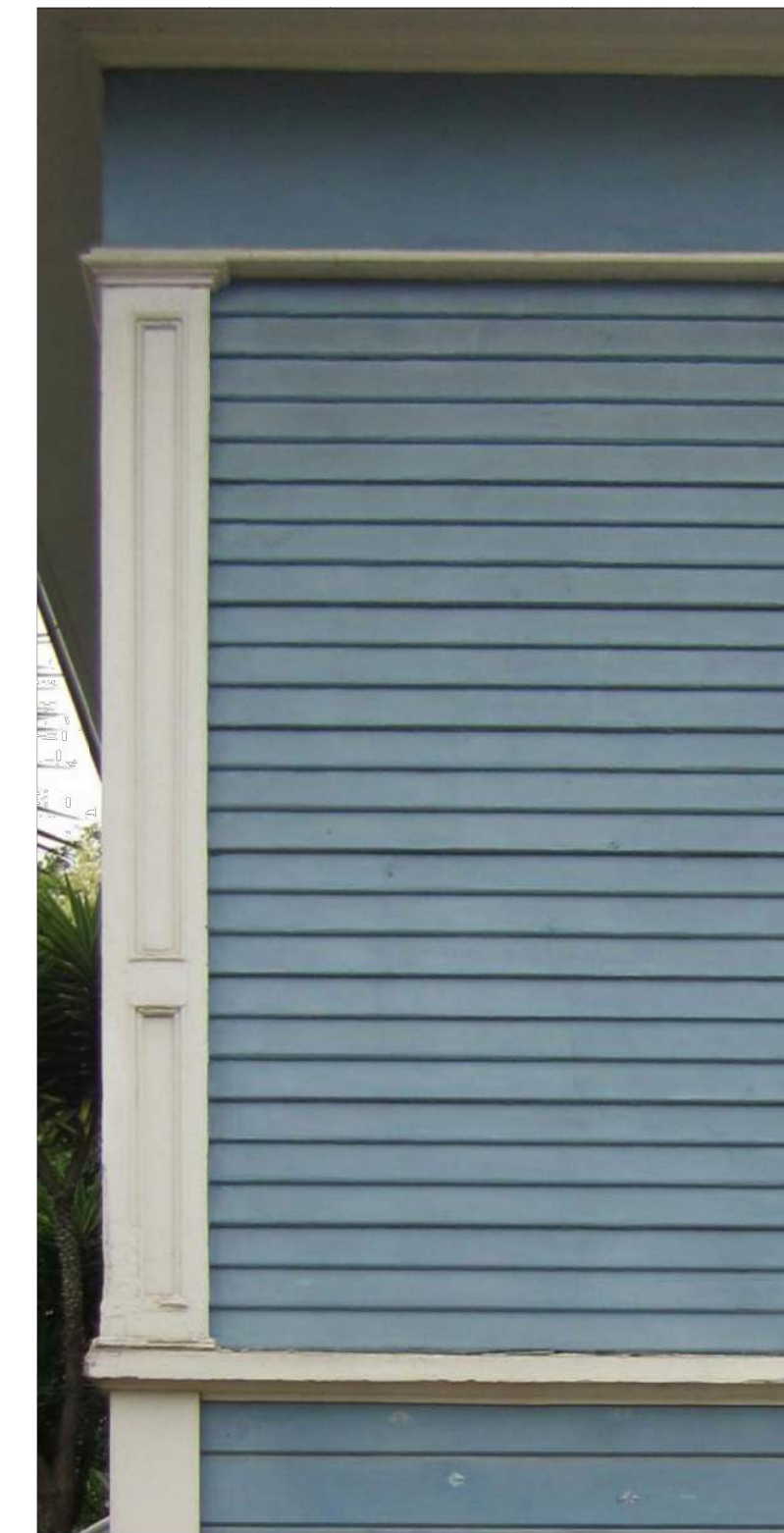
IMAGE: 850 SAN VICENTE - FRIEZE, CLAPBOARD SIDING, STRINGLINE, CORNER TRIM. SAMPLE IMAGE OF HISTORICAL DETAILS TO BE RETAINED
