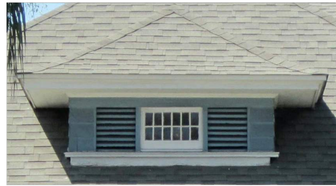
IMAGE: 837 SAN VICENTE. SAMPLE IMAGE OF DORMER VENT DETAILING TO BE RETAINED
