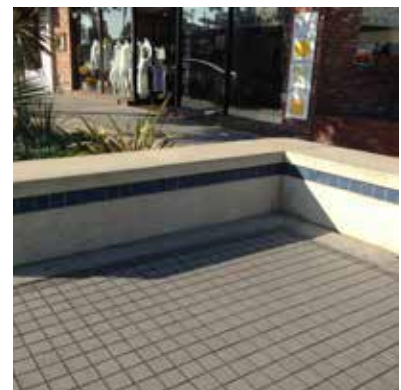
-F3 The concrete benches are worn and the inlay tile motif will need to be replaced to update this outdated look
