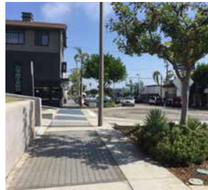
-W9 Although the tile walkways provide a consistent design statement, they have created maintenance issues as well.
