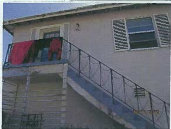
Older multi-family building showing signs of disrepair.
