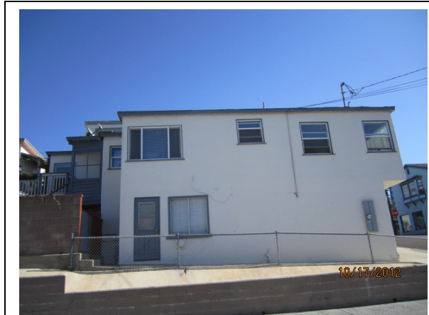
Older underutilized multi-family building showing signs of disrepair and functional obsolescence.
