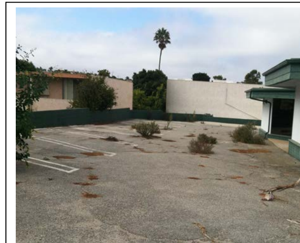
Vacant commercial property with significant deterioration.
