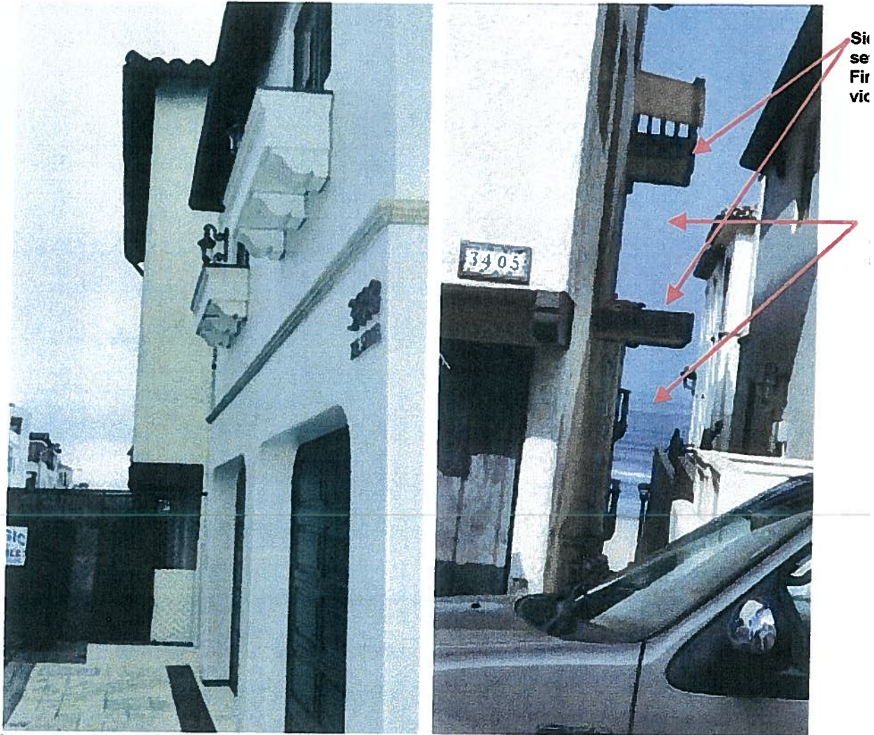
Views of 3405 Ocean Drive projection into front (east) yard and remaining landings where illegal stairs were removed.
