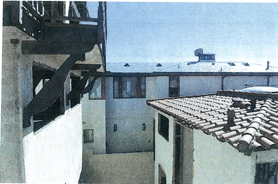
3405 Ocean Drive 3 rd story (directly above garages, below the 4 th story) is at the same height as the adjacent properties' buildings top floors and has an open view over the top of the 3404 The Strand structure.
