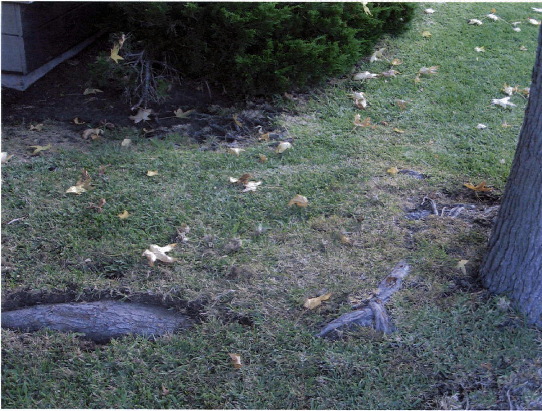
Another view of the large root that heads toward the house's southern wall.
