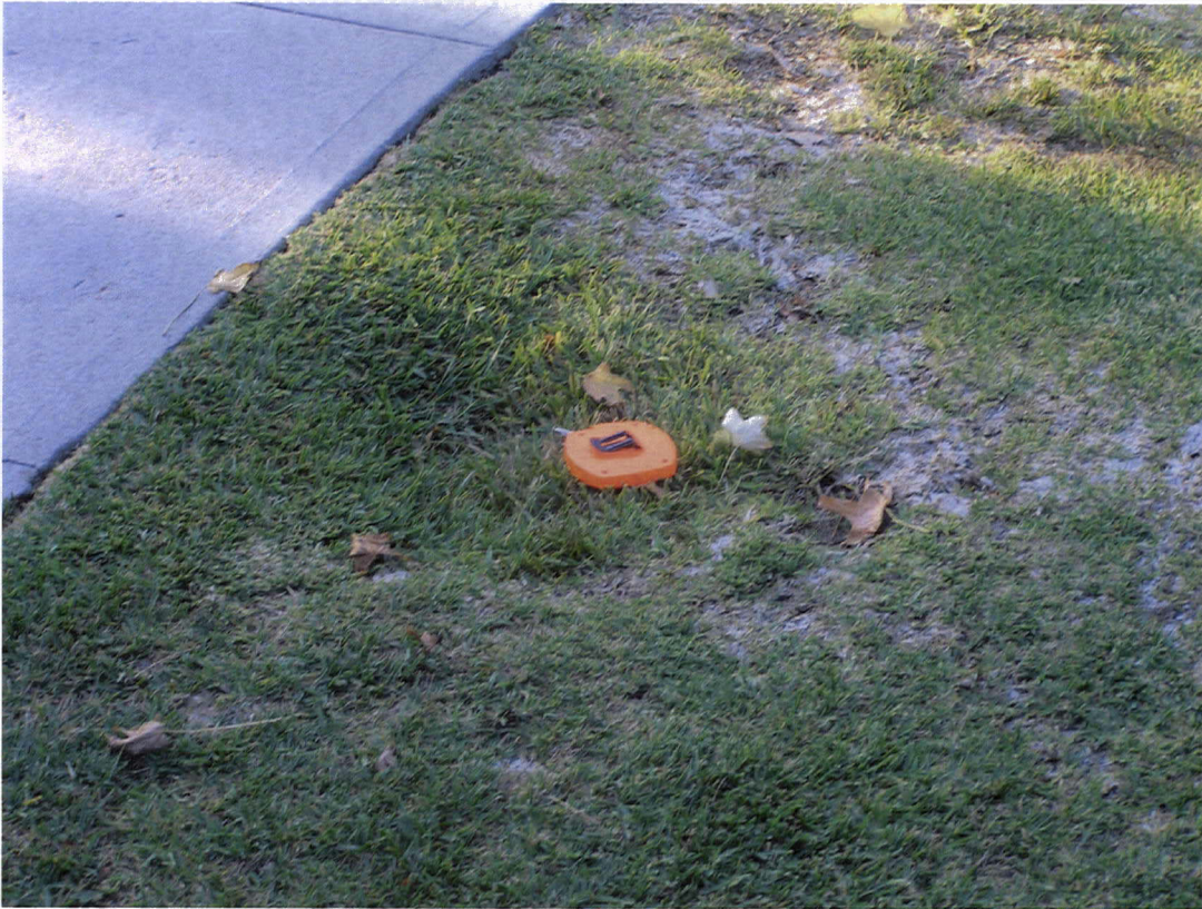
The measuring tape sits on top of a sink hole. The contractor thinks this is the access point for the cesspool.
