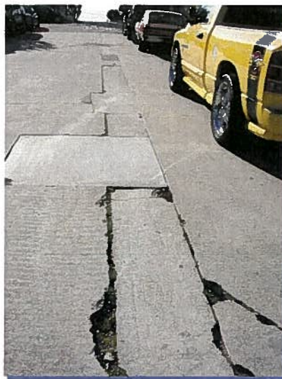
Portion of 7 th St. (not on walk street) water main trench location and surface failure.
