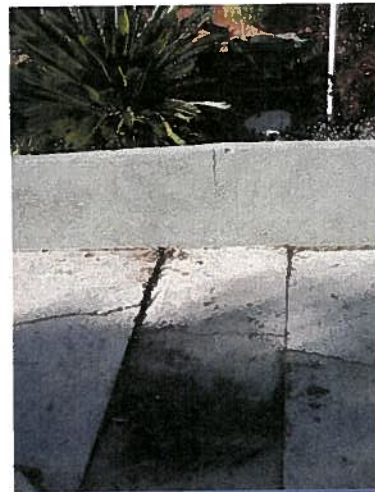
Water meter location and service line trench failure at main.
