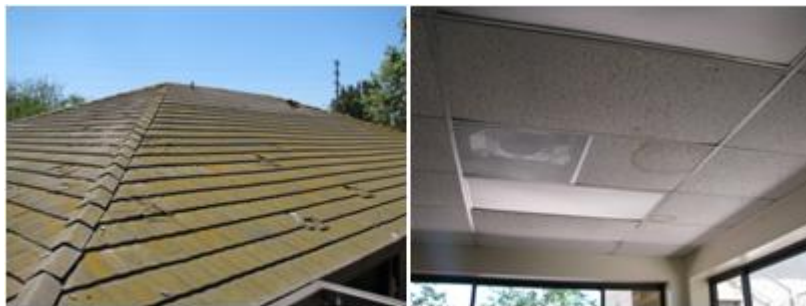
Roof Leaks due to Baseballs
