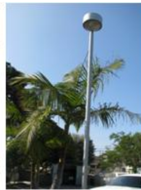
Parking Lot Lighting
