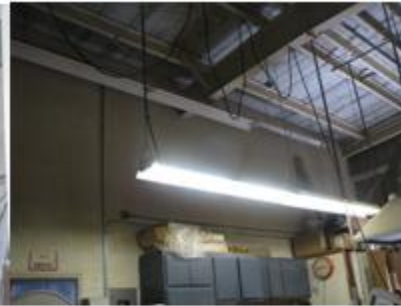
Suspended 8' T8 Fixtures
