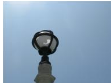
Damaged Pier Globe Lights
