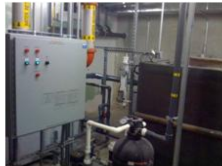
City Hall Mechanical Room
