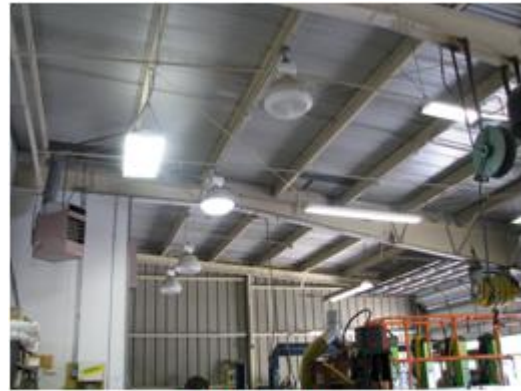
Sample Fixtures 250W Mercury Vapor and T5 Fixtures
