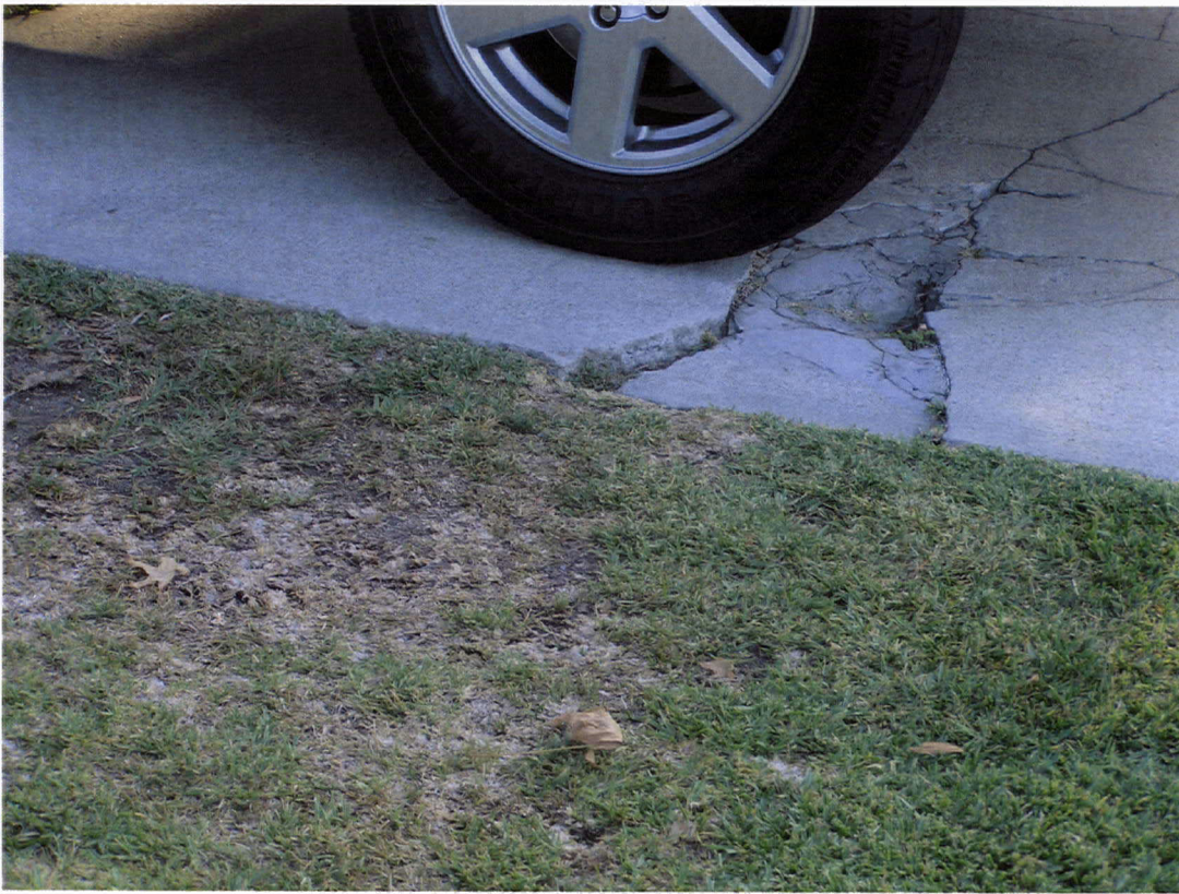
A driveway crack presumably caused by the Liquidambar's roots, 15' east of the tree.
