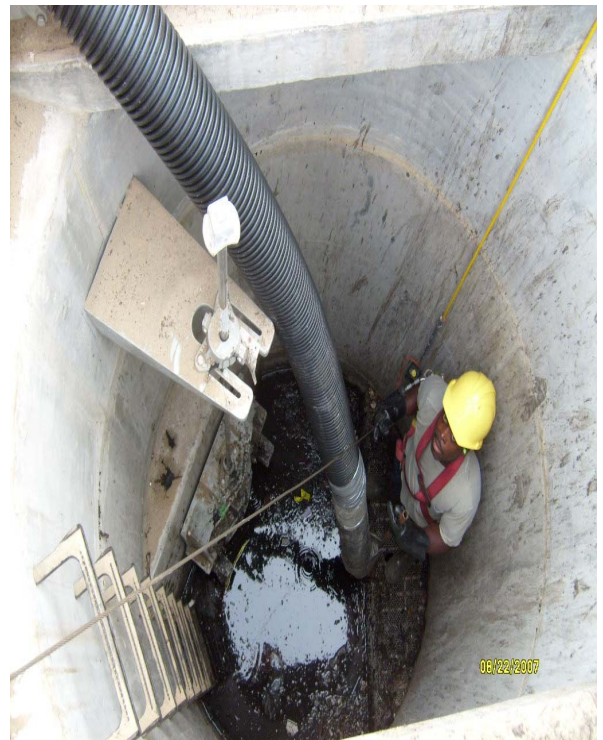
Figure 2 – Maintenance worker working in LFD Structure
