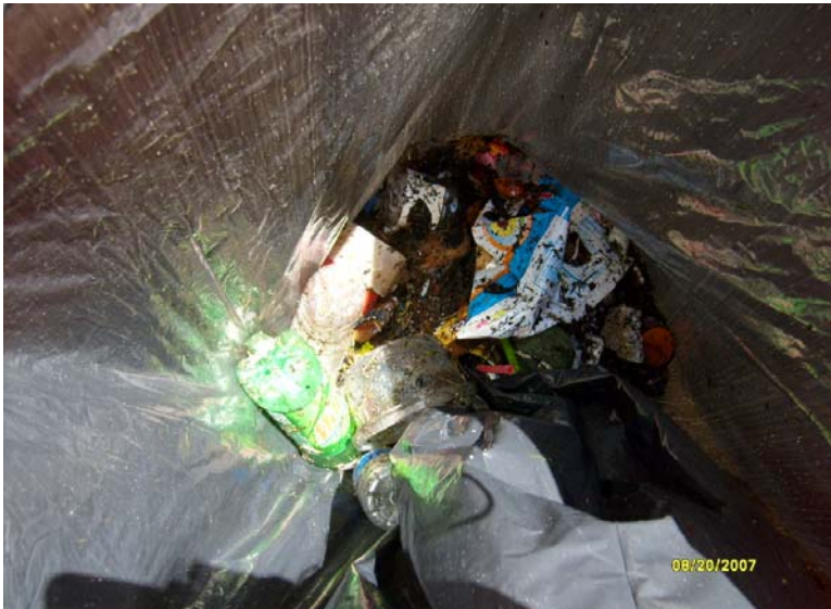
Figure 1 – Trash and Debris caught by Low Flow Diversion Structure
