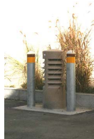
Example of an Above Ground Vent Pipe
