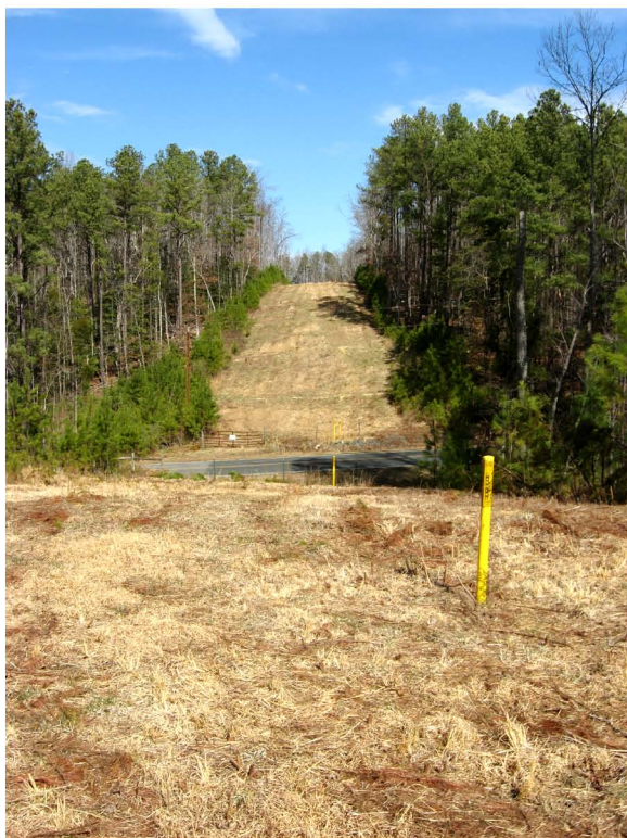
▲ Cardinal right-of-way (R-O-W) crosses Andrews Store Road (center gray line). Lots 19 & 20 (left of R-O-W). Open space (right of R-O-W).
